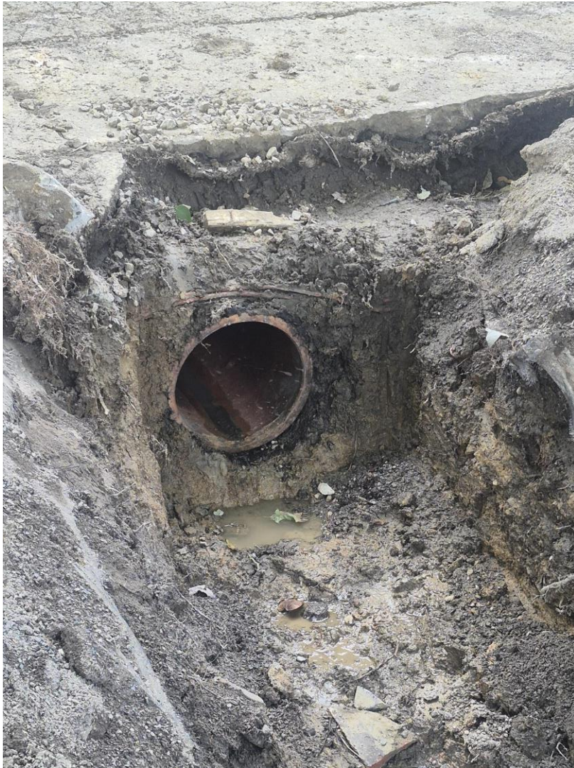
Exposed storm drainpipe
