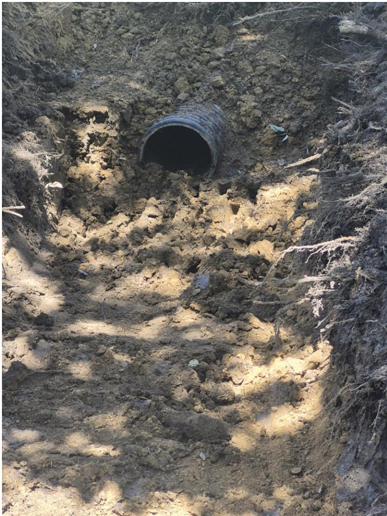
Impacted drain inlet (downstream)
