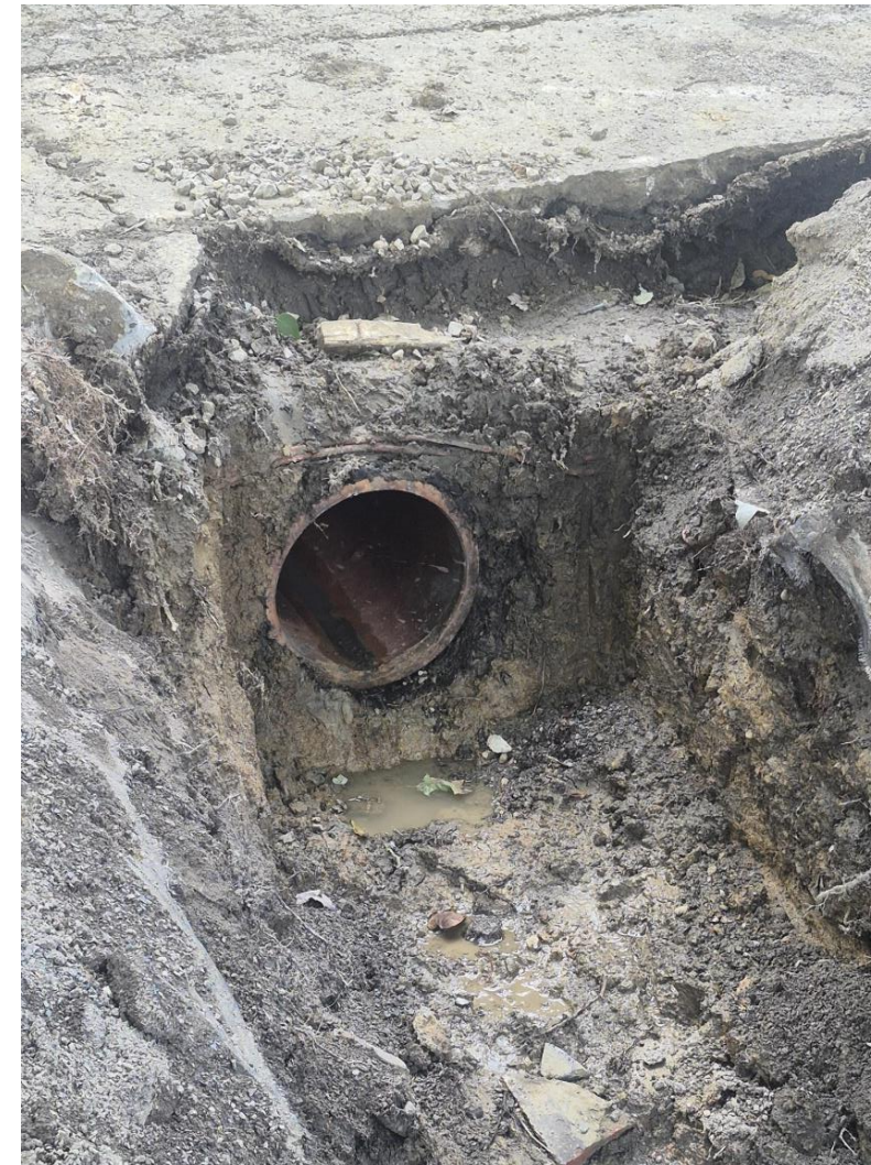
Impacted drain inlet (upstream)
