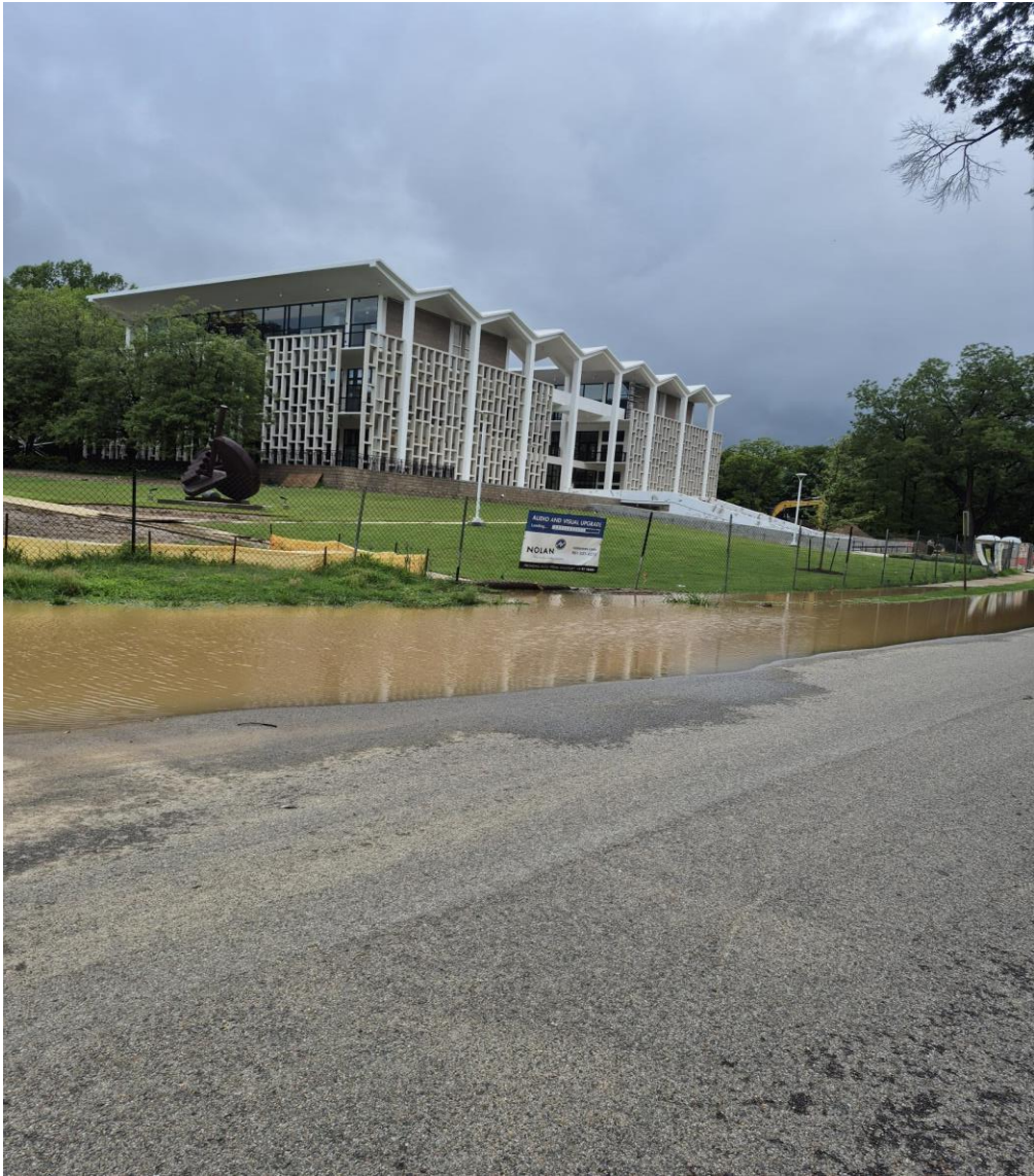
Water pooling, cont'd.
