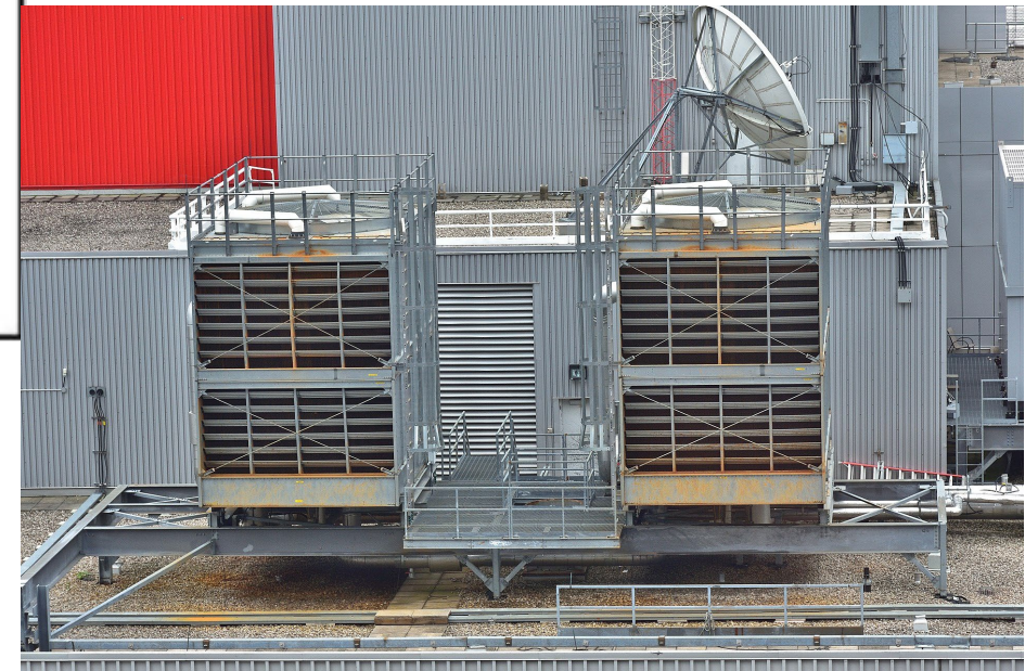
Evaporative cooling tower
